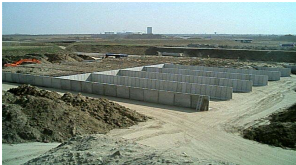
Figure 11: EK remediation plant during first loading. Each bay measuring 10 x 30 x 3 metres has a capacity of 2,000 tons
